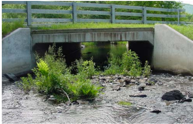
Figure 7.2.3 Deposition at the upstream end of the box culvert located on River Street.
