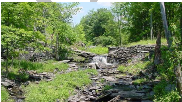
Figure 7.2.2 Remains of the old mill dam located approximately 375 feet upstream from River Street stone arch bridge.
