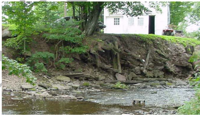
Figure 7.3.13 Looking downstream at an eroding bank located approximately 1,750 feet upstream from County Bridge 18-6.
