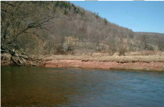
Figure 7.3. 15 An eroding bank downstream of railroad bridge where bank pin #34.3 is located.
