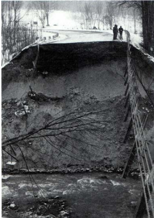
Figure 5.7 Washout on Chase Brook Road over Chase Brook near Cannonsville Reservoir, January 19, 1996
