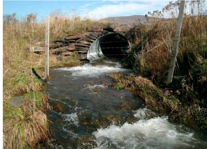
Figure 2.3 Culvert installation that could benefit from improved alignment, fish passage, outfall dissipation, headwall installation and top cover.
