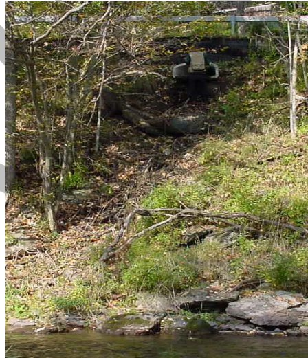
Figure 2.1 Poorly designed culvert outfall along NYS Route 10 upstream of Bloomville. Note direct discharge into river with lack of energy dissipation and sediment control measures. This site could benefit from a stormwater retrofit.
