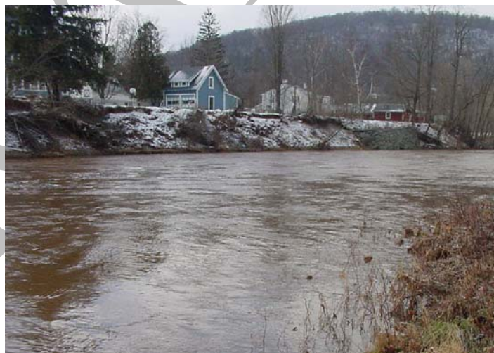
South Street location showing condition of embankment (December, 2000).
