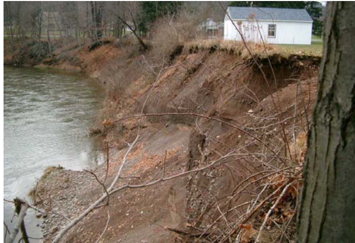
Closer view of the unstable embankment at the Terrace Avenue site (December, 2004).
